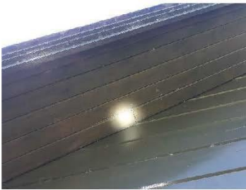
Loose Soffit Boards, Potential Bat Roosting Feature
