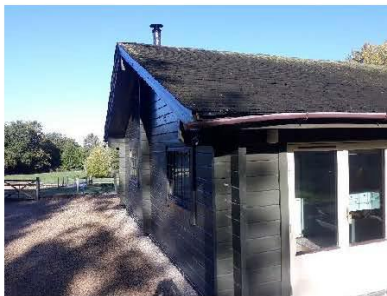
Loose guttering access to roof space, Potential Bat roost feature
